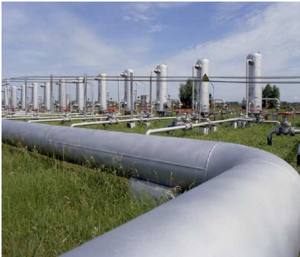
Natural gas (methane) pipeline.
